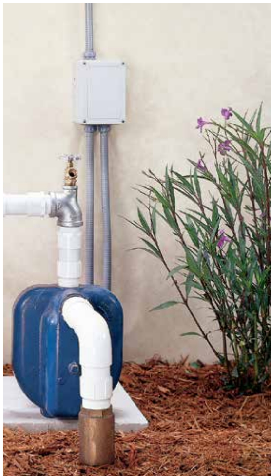
pump start relays
